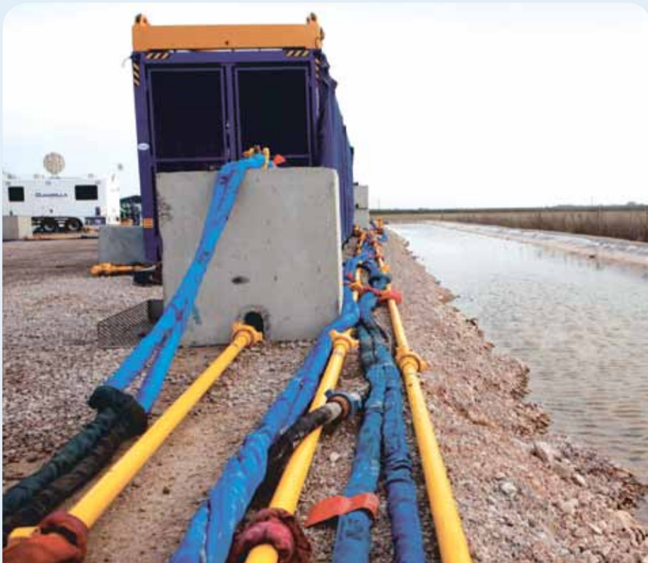
The impermeable membrane runs under the site and prevents any potential spills from leaching directly into the groundwater.
